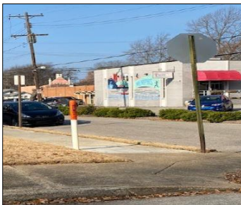
Figure 6.1: Unacceptable Fiber Route Marker
