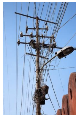
Figure 2.4: Unacceptable Strand Mount
