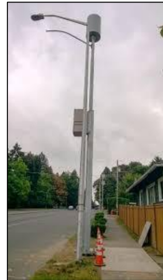
Figure 5. 1: Freestanding Pole adjacent to existing light pole.
